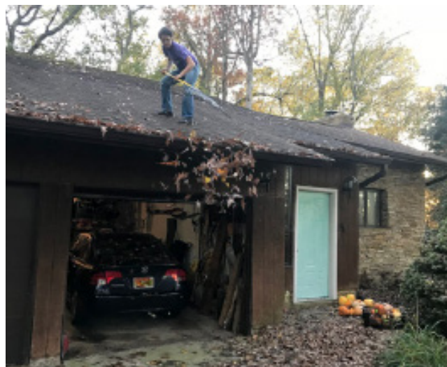
After recent rains, it became necessary to rake leaves off of this roof
