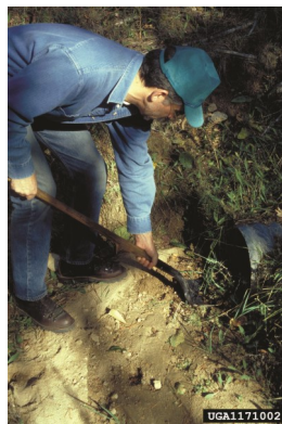
Cleaning out trail or road culverts is an essential BMP. Photo courtesy Chris Schnepf, University of Idaho, www.forestryimages.org
